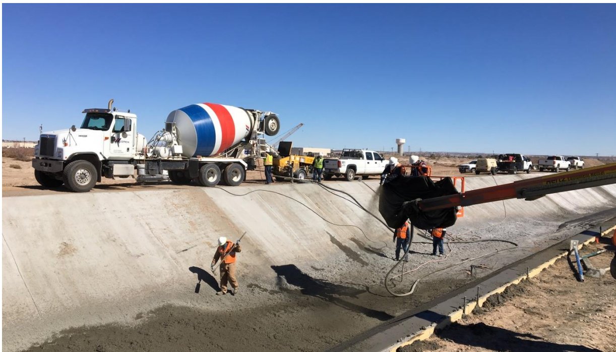
Figure 10. Canal lining funded through the El Paso County Water Improvement District No. 1.
