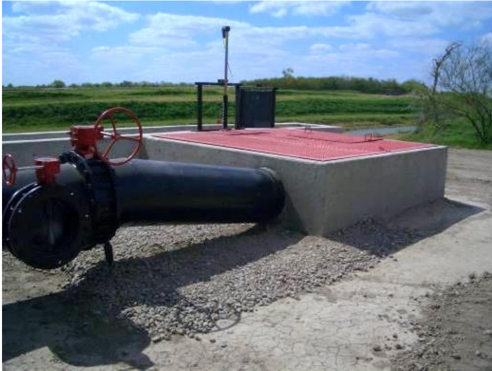
Manifold discharge and calibration tank.
