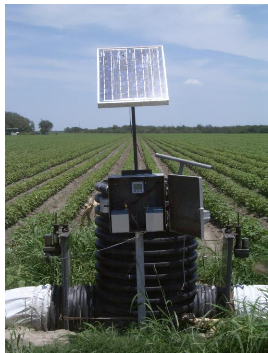
Surge valve with solar-powered controller.
