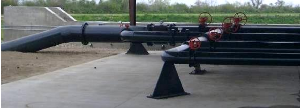
Closed pipe manifold.
