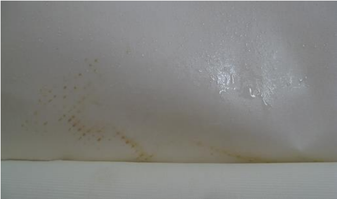
Figure 8. Close-up of the membrane backing material from element F5375550.
