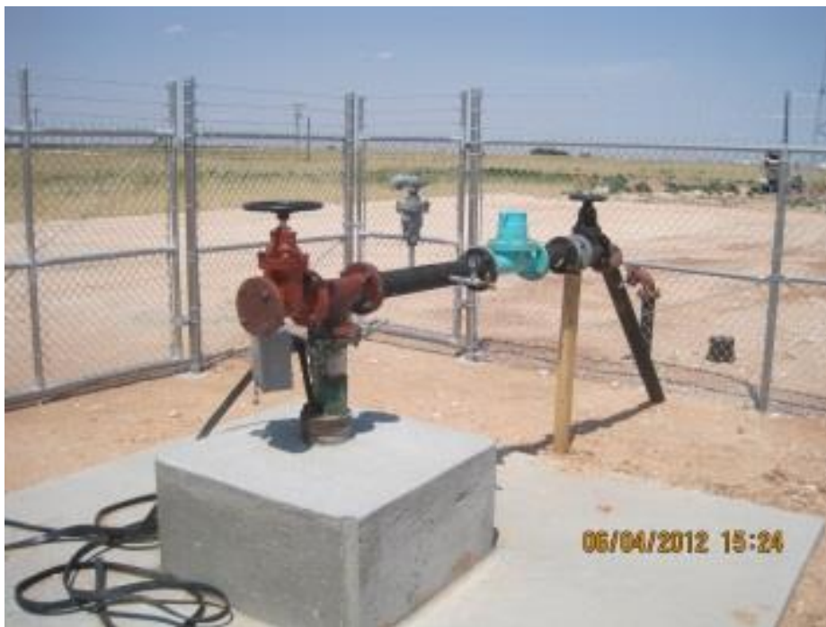
Figure 5. Complete well and plumbing
