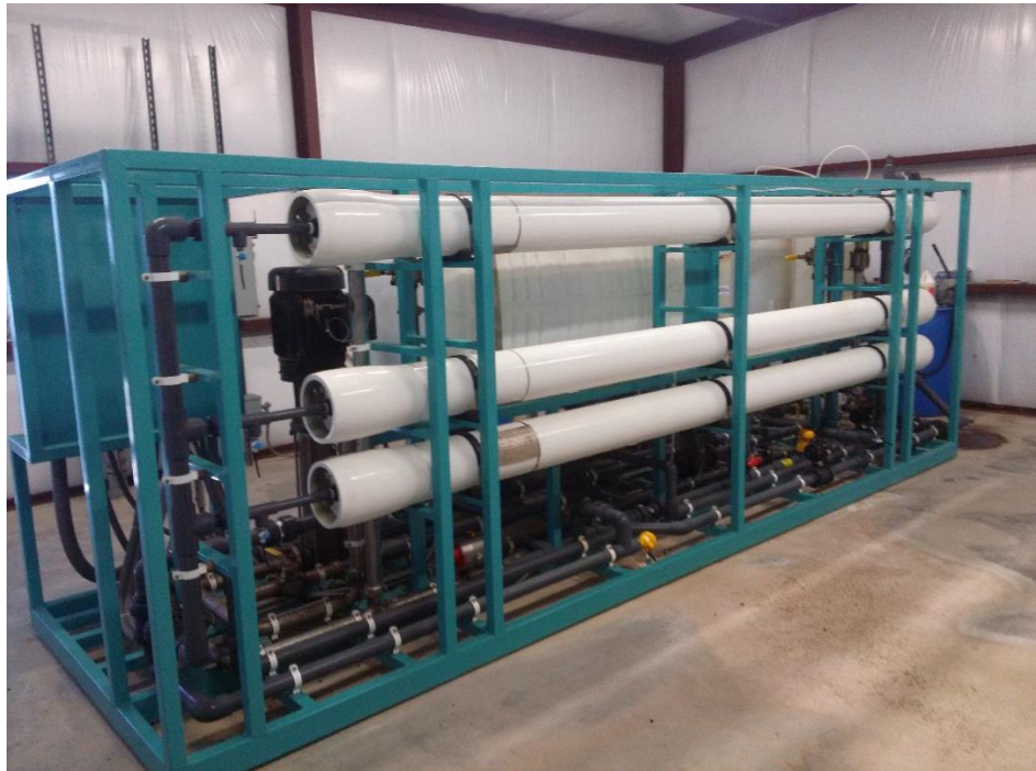
Figure 8. RO skid in place at the demonstration site
