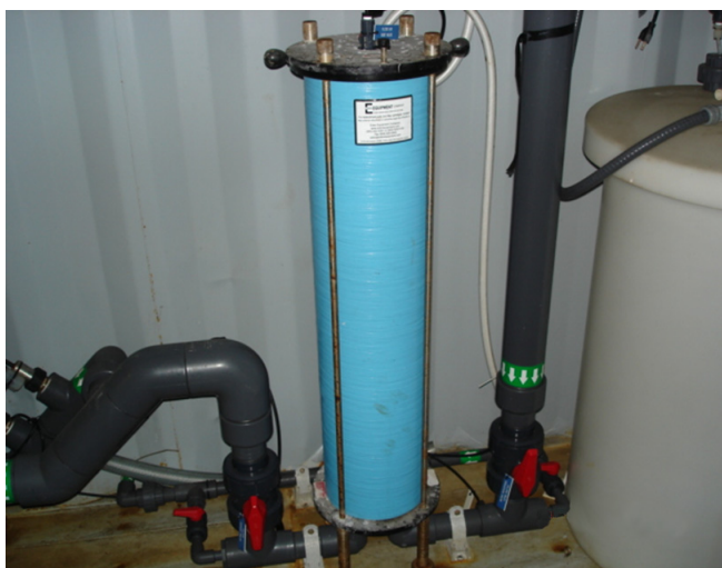
Figure II-15: Cartridge filter housing mounted inside RO container.
