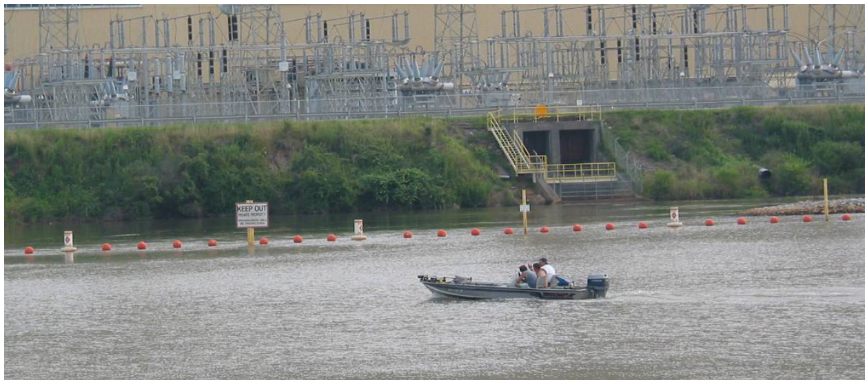
Figure I-15: An exclusion system, demarcated by red floats, at a power plant on Lake Sinclair, near Milledgeville, Georgia
