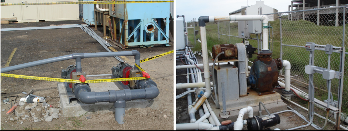
Figure II-7: Original intake pump system (left), most recent intake pump (right).
