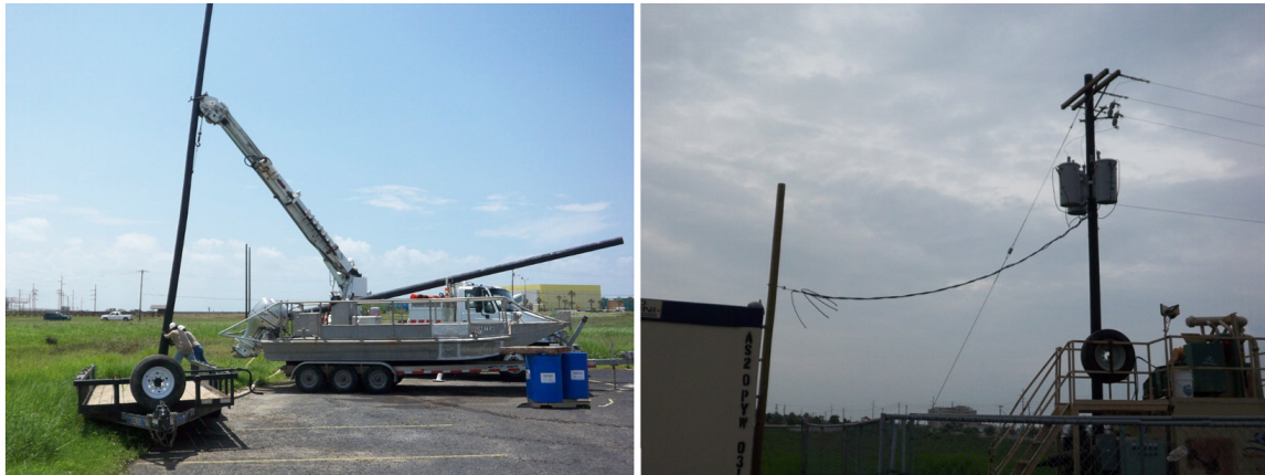
Figure II-3: AEP installing distribution line (left), three phase power installation completed by AEP (right).
