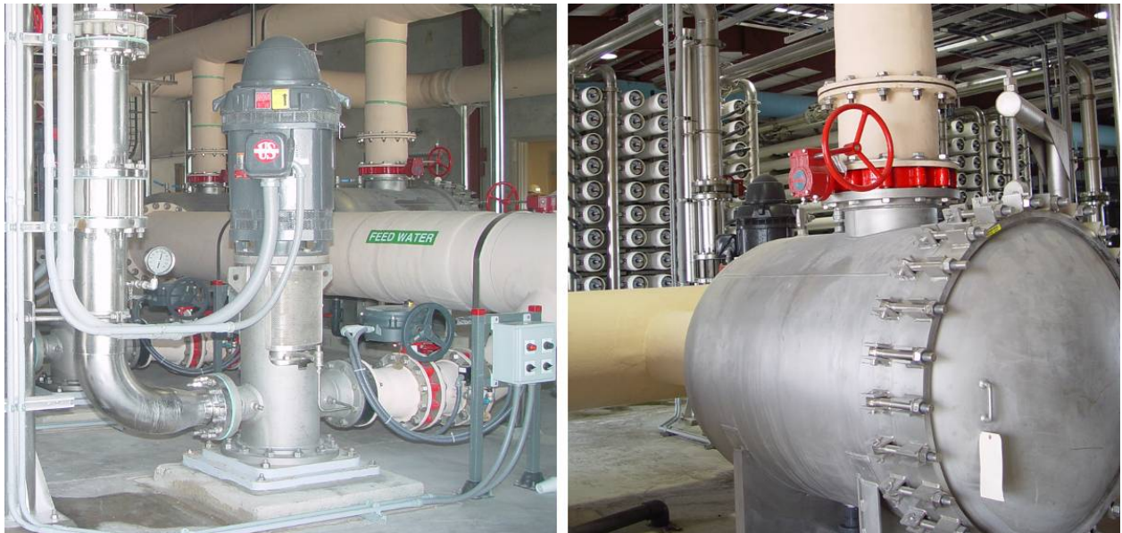
Figure I-40: Southmost Regional Water Authority brackish desalination plant high pressure RO feed pump (left) and cartridge filter (right).
