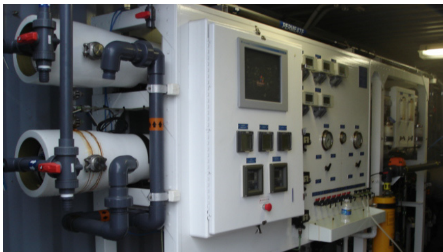
Figure II-13: RO pressure vessels and control panel.
