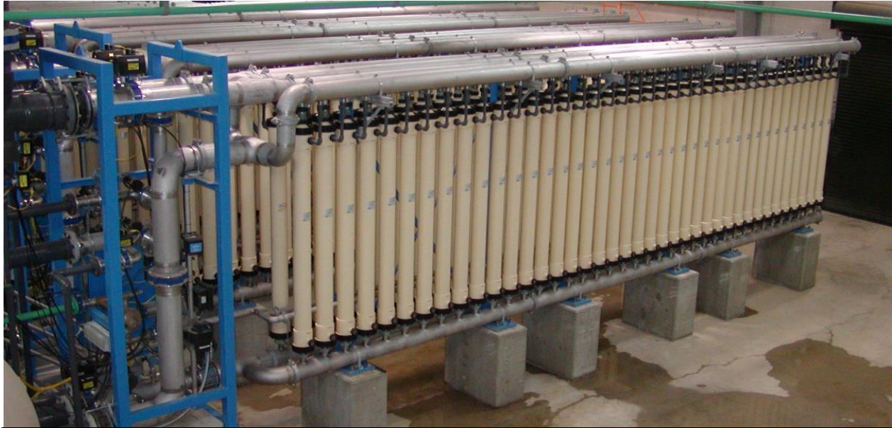
Figure I-39: Pall MF System in Temple, Texas.
