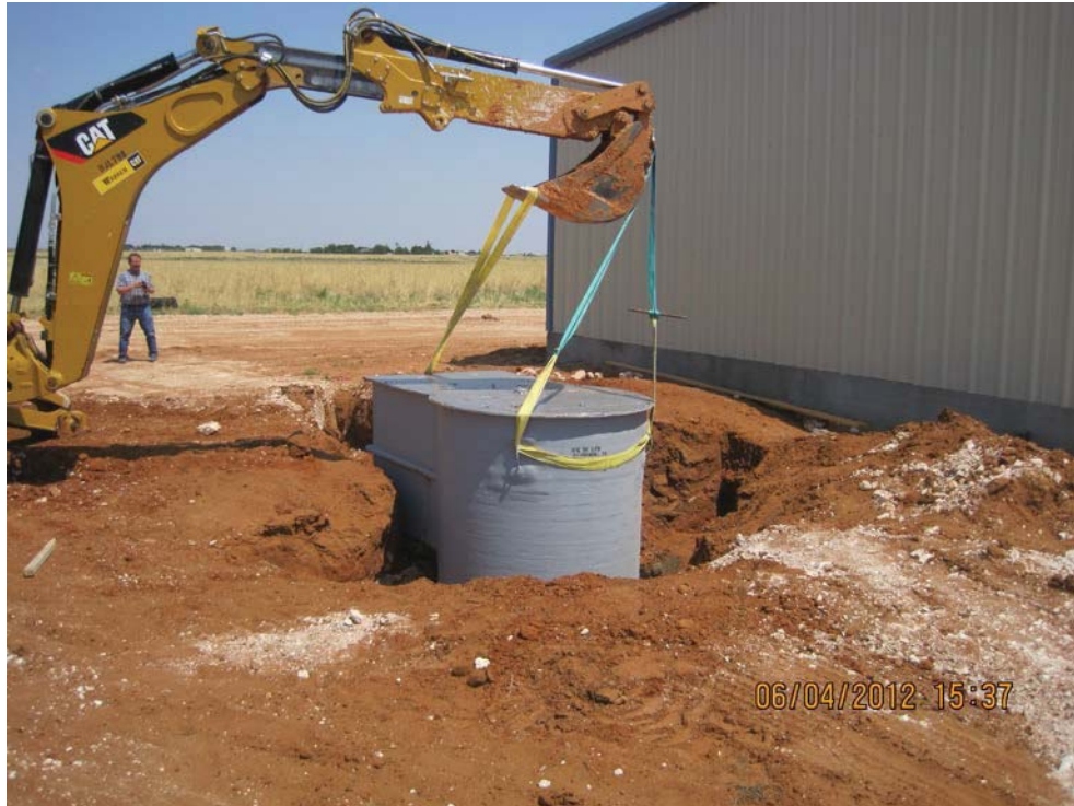
Figure 3. Lift station north of RO building
