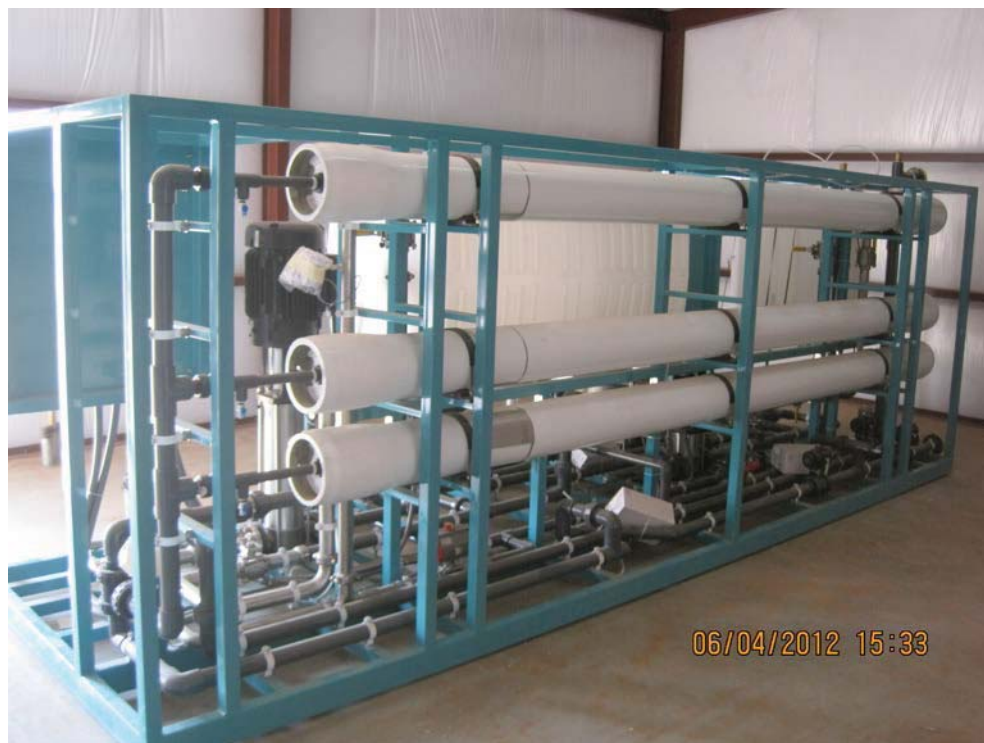
Figure 2. RO system inside RO building
