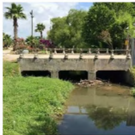
Figure 2-3: Culvert blockage under Access Road 1 upstream of Sunny Flea Market
